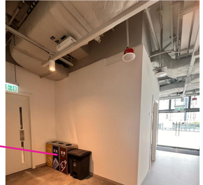
Next to the smoke stop door, CityUHK International Centre
